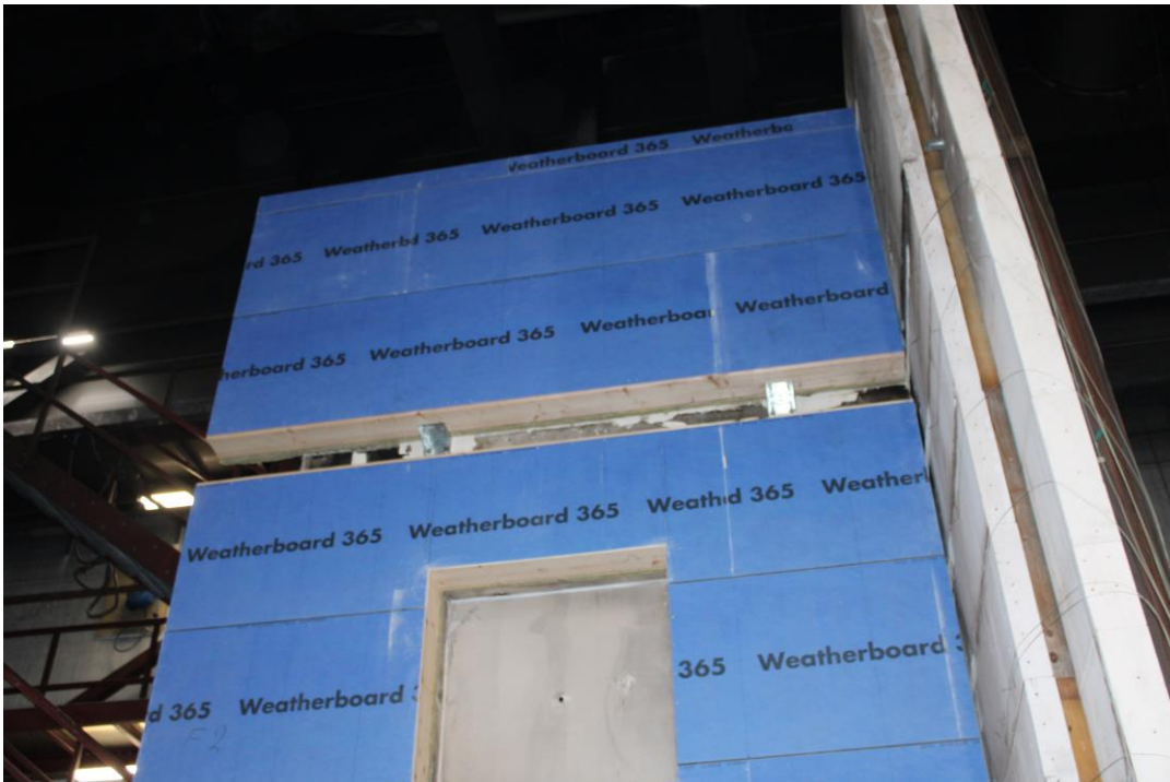
Photo No. 2 The prefabricated cassettes was mounted with steel brackets, leaving a gap.
