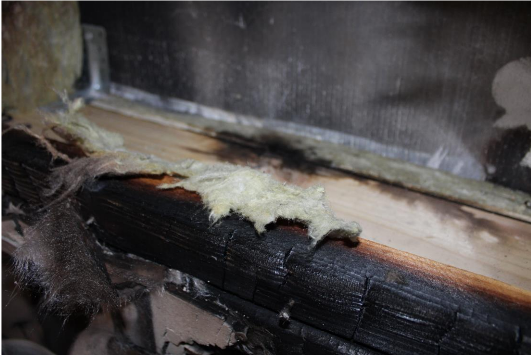
Photo No. 25 Test specimen after the test. Detailed photo of wooden frame
