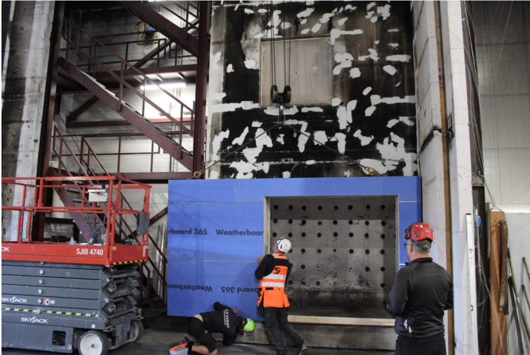
Photo No. 1 Prefabricated cassettes were mounted to the aerated concrete with stone wool in between the cassette and the concrete.
