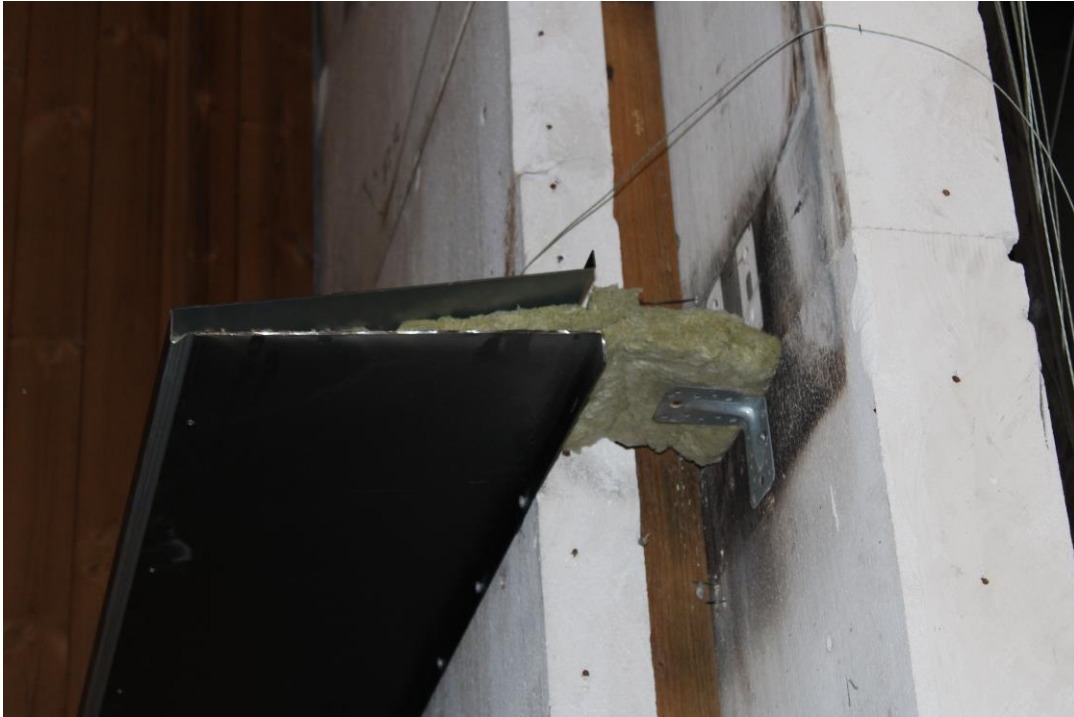
Photo No. 9 The ends of the flame deflector was closed off with stone wool.
