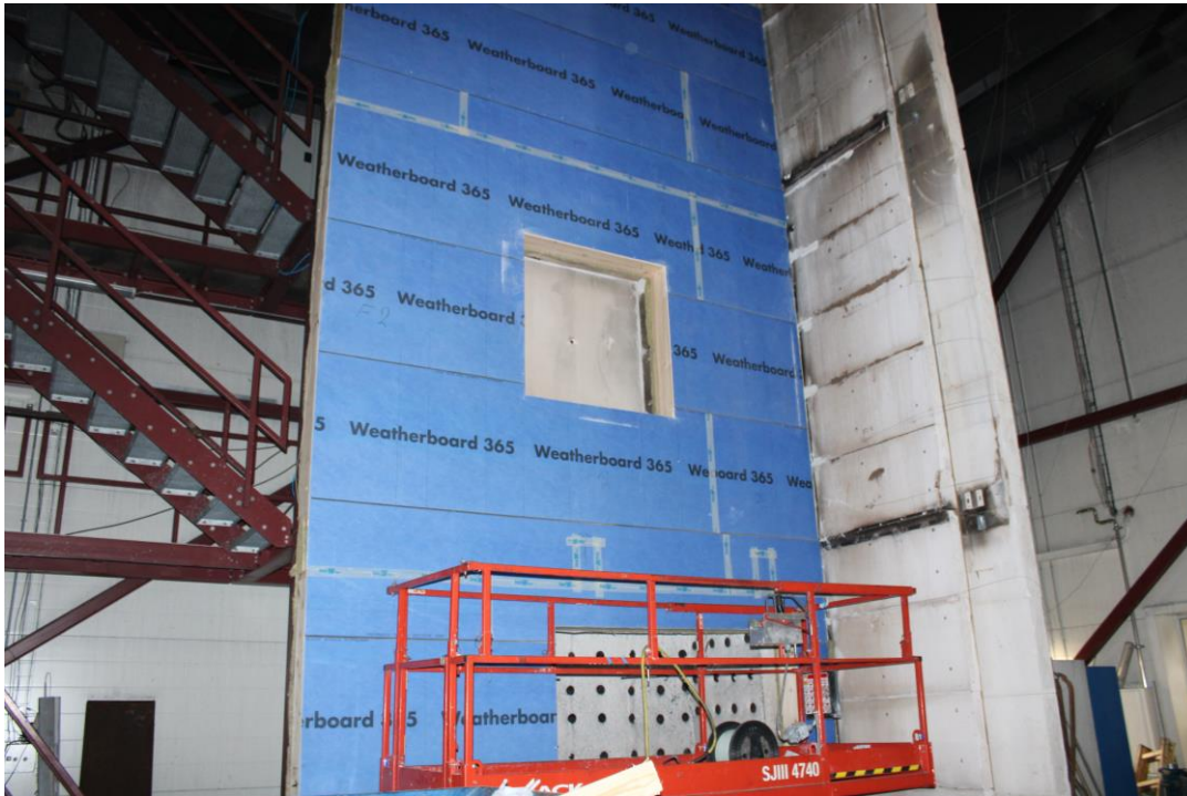
Photo No. 3 The vertical gaps was closed off with rockwool and weatherboards as seen in the picture.
